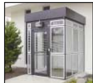
Three-sided vestibule with magnetic locks
